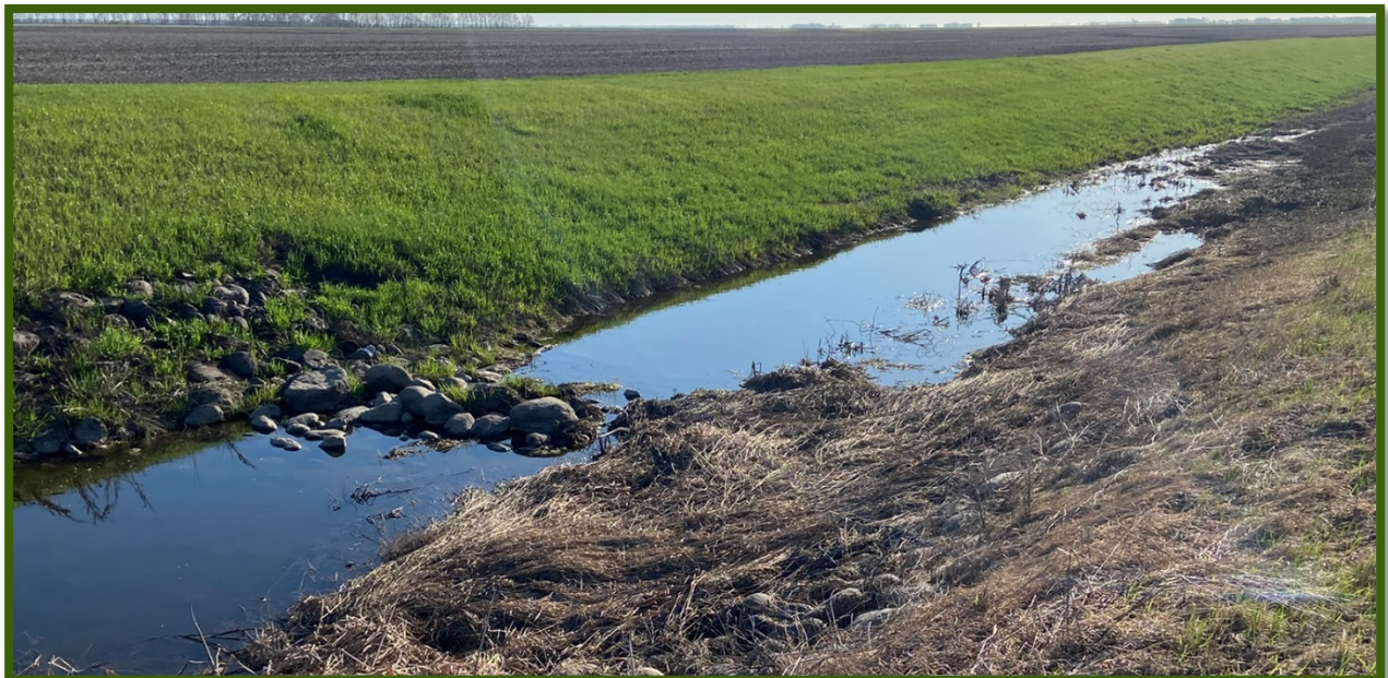
Exhibit 2 - Drain 4 Downstream Scour Hole
