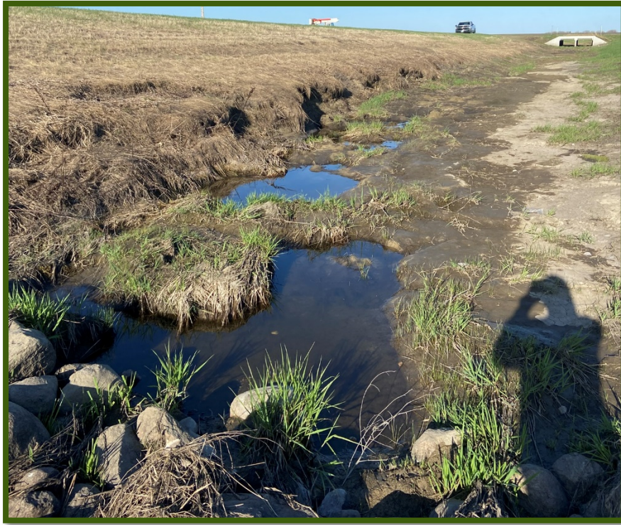
Exhibit 1 - Drain 4 Bank Failure
